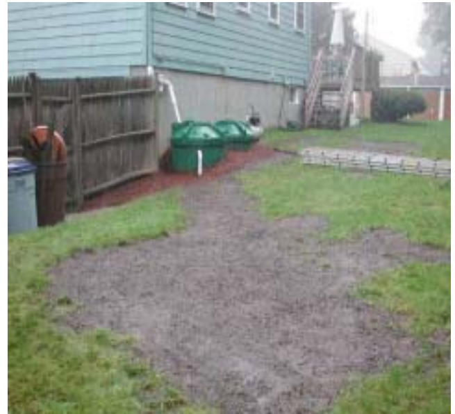
Manufactured dry well system after installation. The dirt areas indicate where the well was buried. The green objects are storage tanks with a pump. Drywells also work well receiving rain barrel overflow (Photo: Charles River Watershed Association)
