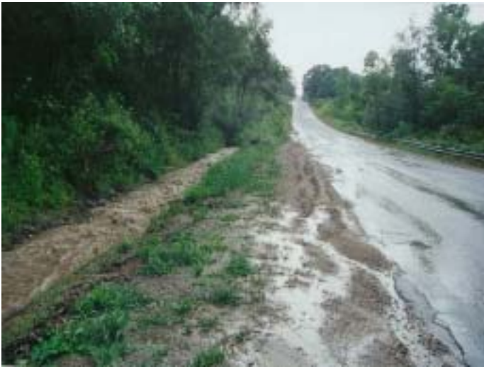
Roadside erosion due to flooding (Photo: Patricia Pennel)
