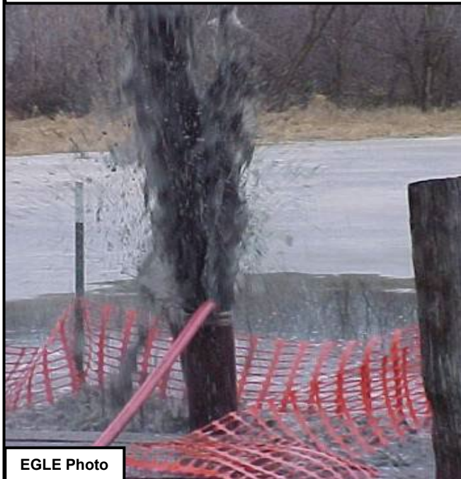
Surging sediment and debris out of an abandoned water well in Jackson County, Michigan
