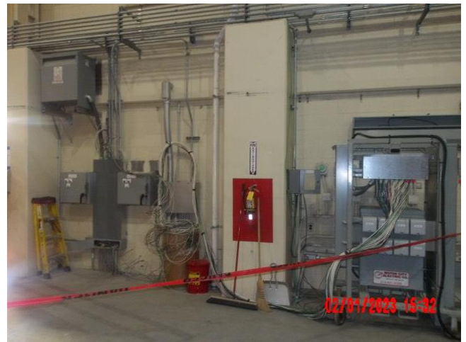
New Lighting Panel D with new Transformer on first floor
