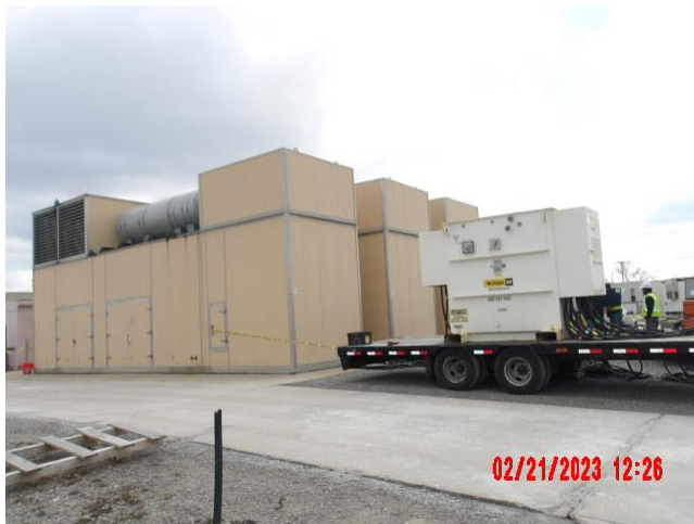
PM Technologies conducting over-stress test for electrical generators
