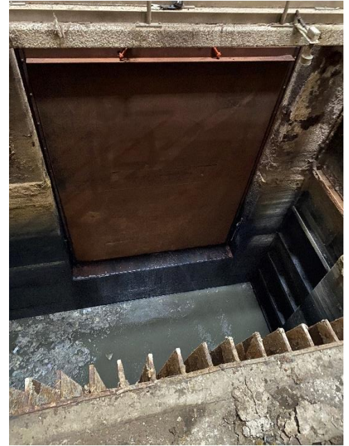
Minimal leakage around OMIDDD Interceptor after stop log installation
