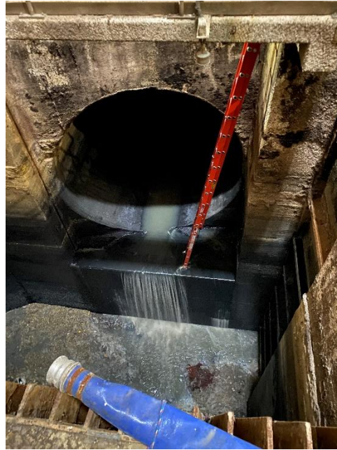
OMIDDD Interceptor with some sewage leaking while CS-9 is closed
