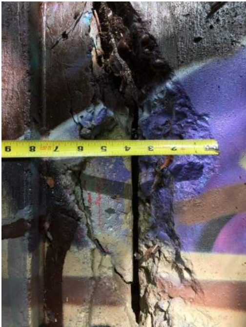
Picture 16: Width of Spall
