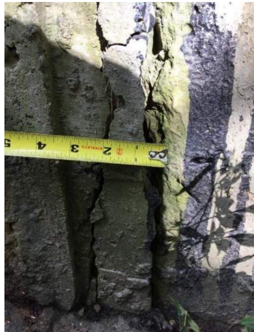
Picture 17: Width of Joint Opening at Bottom
