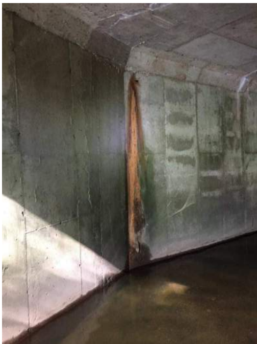
Picture 13: Staining Within Junction Chamber; East Chamber
