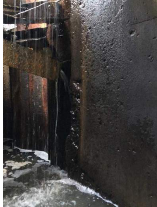
Picture 12: Junction Chamber Concrete Erosion - Eastern Corner
