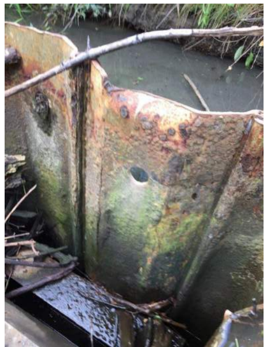
Picture 3: Sheet Pile Corrosion
