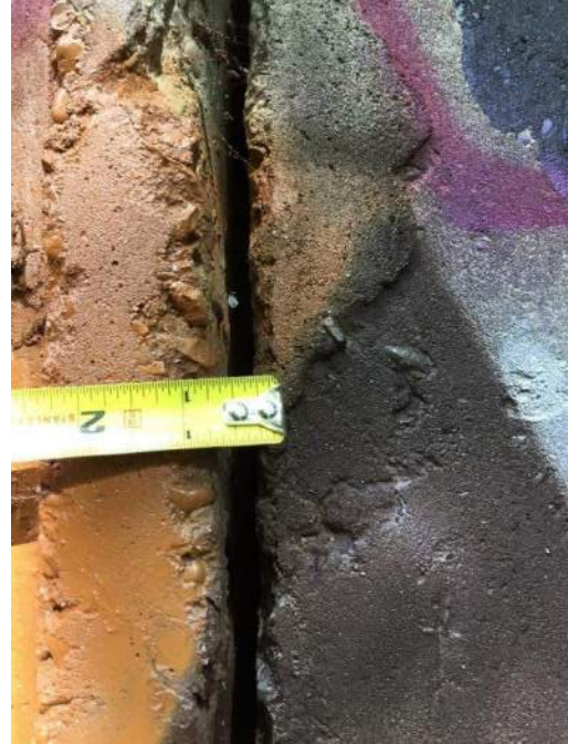
Picture 14: Width of Joint Opening at Top
