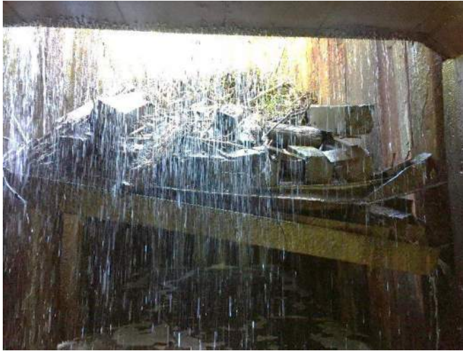
Picture 5: Collapsed Drop Fall Structure as Viewed from Within Junction Chamber
