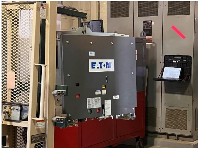
Sanitary Pump #4. Breaker removed for annual cleaning and inspection
