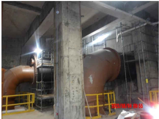
Contractor installing the exterior FRP coat for Pump No. 1 and 2 on August 4, 2023
