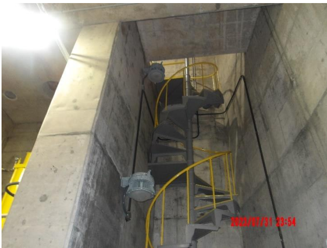
New lighting system for spiral staircase
