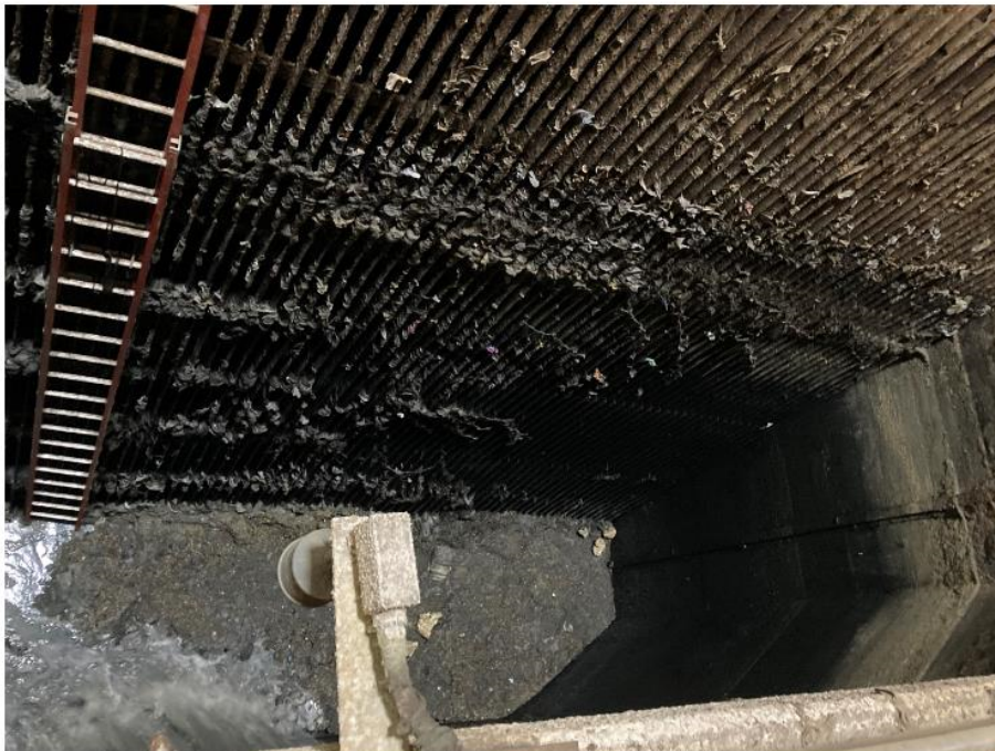
Corridor Chamber Wet Well
