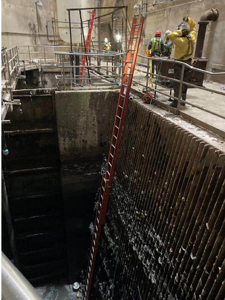
Corridor Chamber Bar Screen
