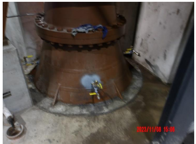
Pressure gauges installed at Pumps #1 and #3
