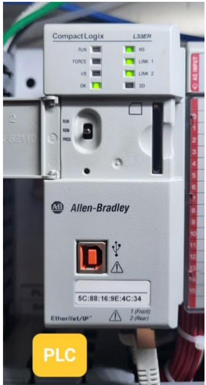
Failed PLC at Bio-filter
