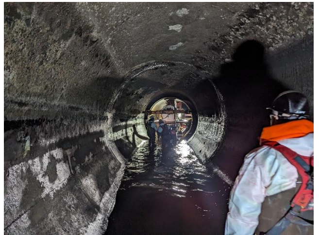
Pipe carrier viewed from inside RAI
