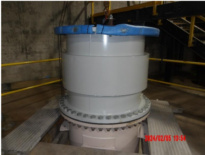
New magnetic flow meter at Pump #5
