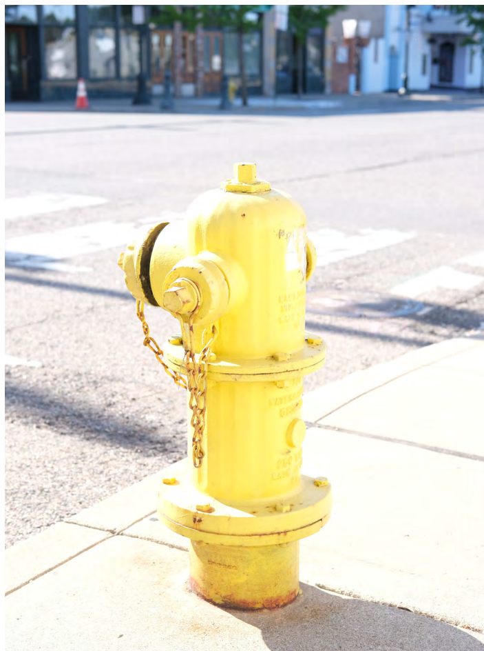
Hydrant, City of Pontiac
