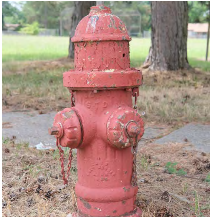
Hydrant , Charter Township of Royal Oak
