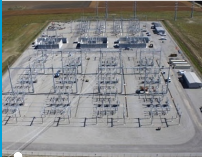
Rapson Substation Huron County
