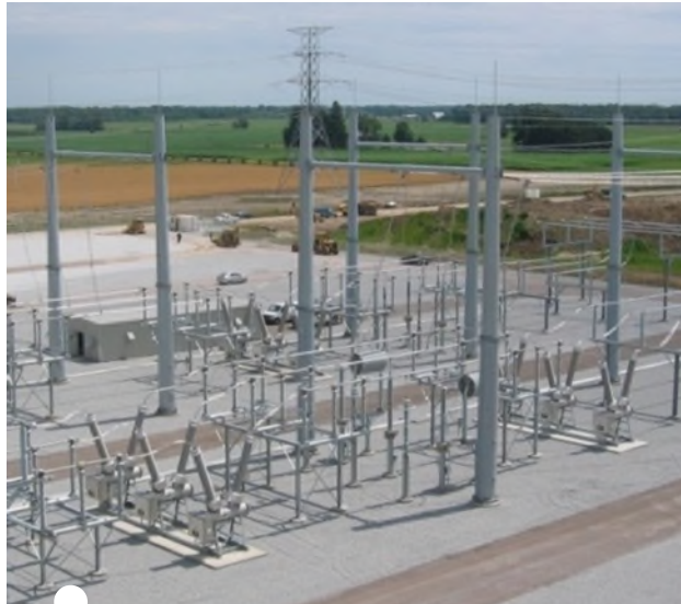
Murphy Substation Saginaw County
