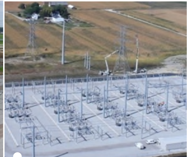
Bauer Substation Tuscola County
