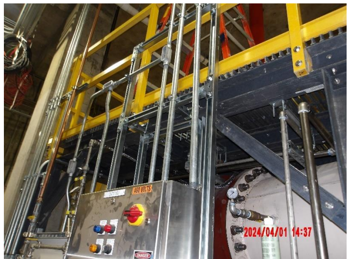
New electrical for Pump #5 lube oil machine and vibration panel
