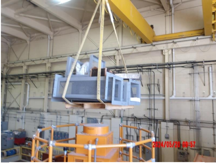
Delivery of 12-inch pump shaft guard
