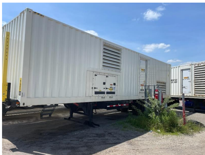
2 Megawatt portable generator unit
