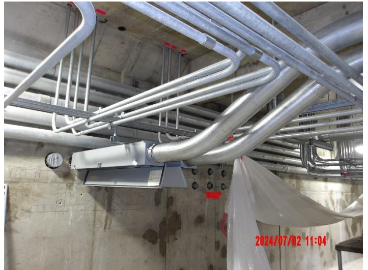
New conduits for high voltage power lines
