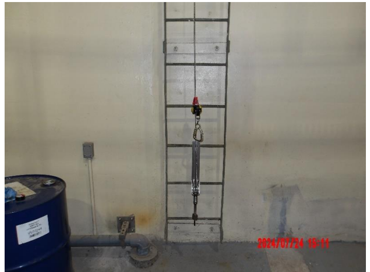
New overhead safety ladder in NESPS
