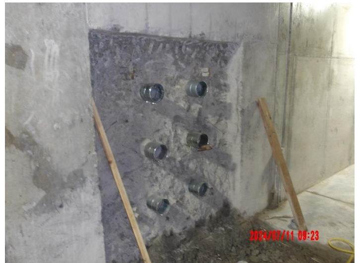
Extension of existing conduits for future use
