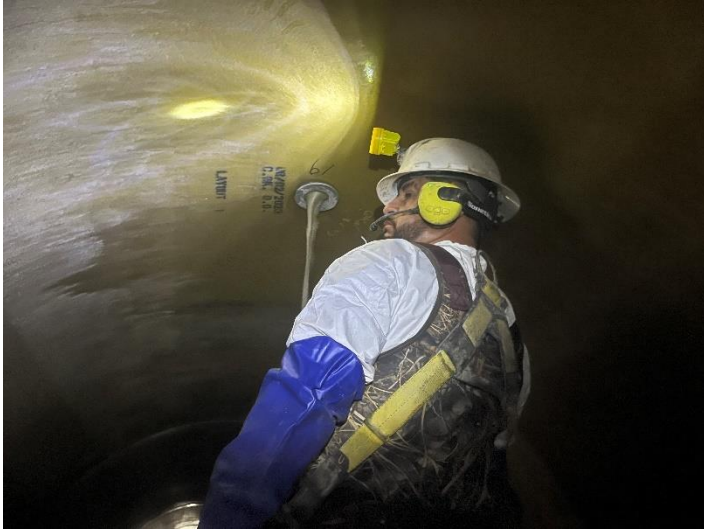
Grout communication at Hobas section 225
