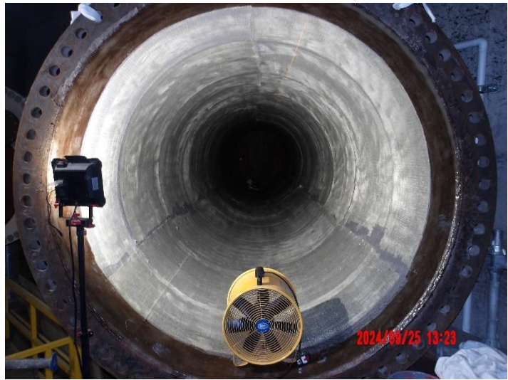
Pump #6 discharge piping interior FRP lining
