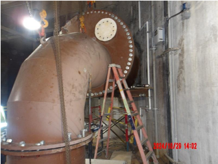
Pump #6 Discharge 90° Elbow
