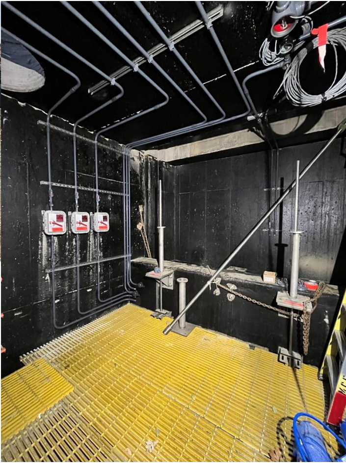
Electrical and Communication installation
