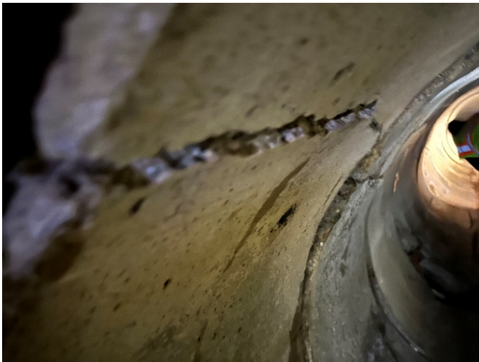
Severed Pipe Sections
