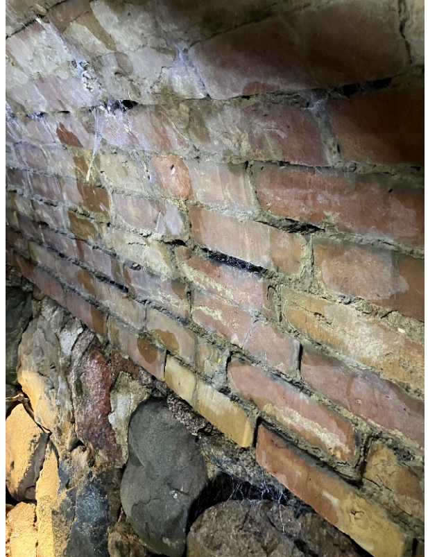
Cracks Within the Brick Arch
