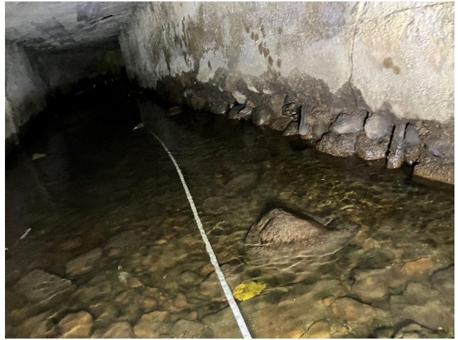
Significant Wall Erosion
