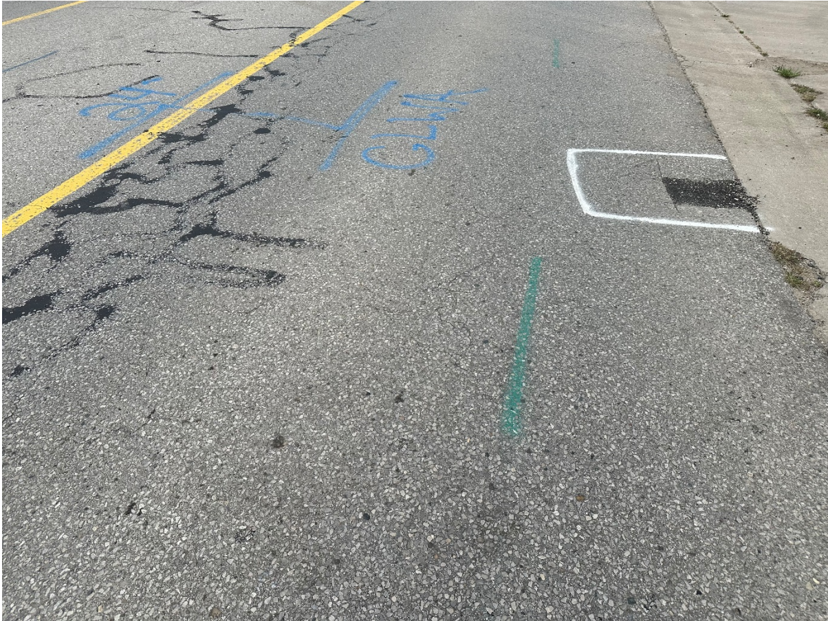
Sink Hole Looking North
