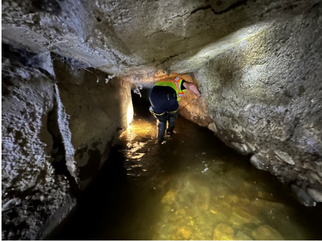
Significant Wall Erosion
