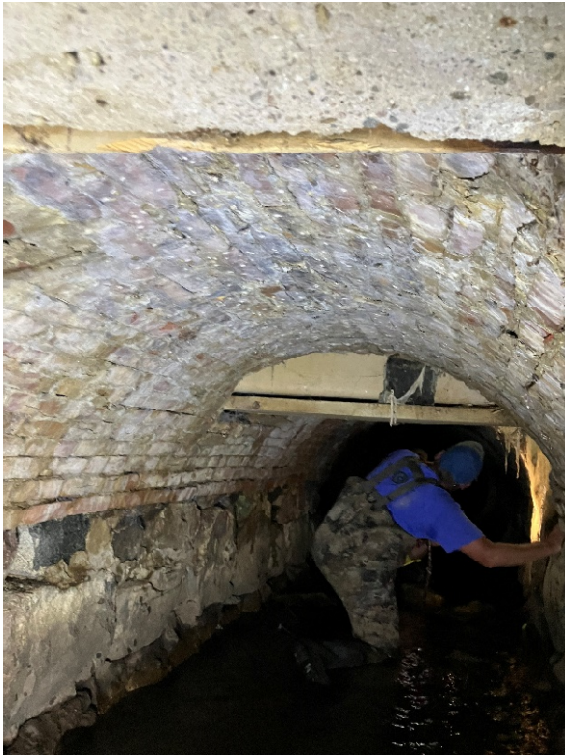
Loss of Mortar Support
