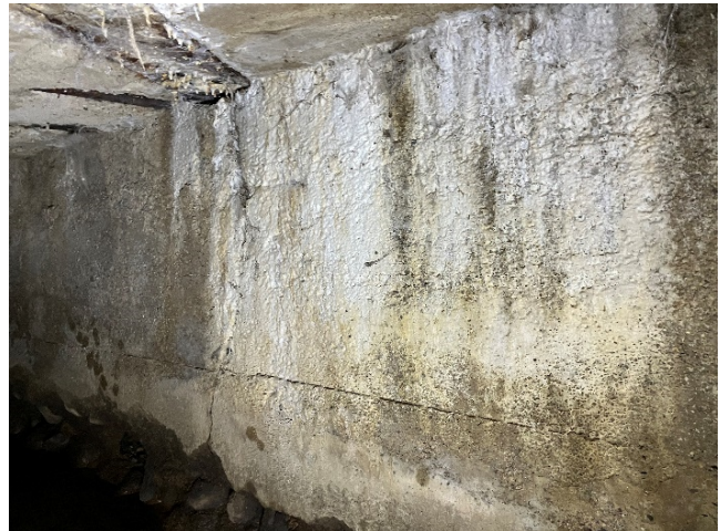
Top Slab Efflorescence
