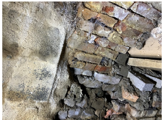
Loss of wall Arch Support
