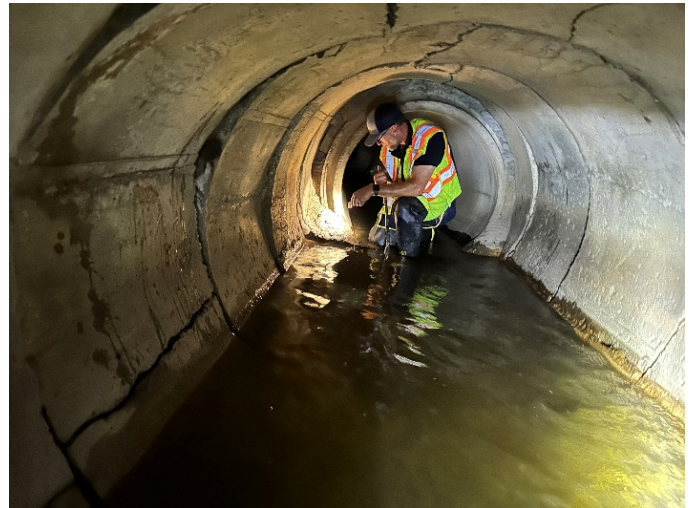
Cracked and Deteriorated Sections
