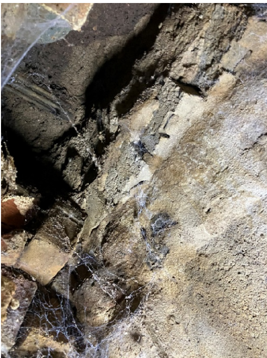
Void in Brick Arch (Looking up)
