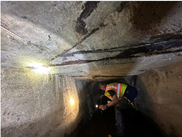
Significant Top Slab Deterioration
