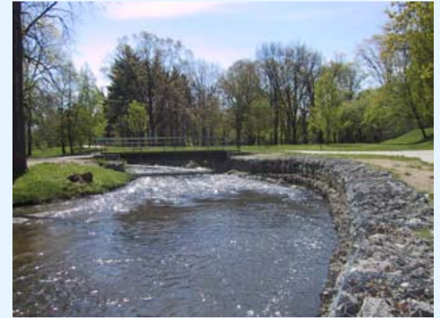
Rock-filled gabion baskets provide stream bank stabilization in the City of Rochester Municipal Park.
