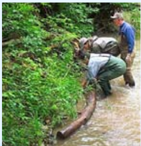
Volunteers help to stabilize an eroding streambank along the Johnson Creek in Northville Township. Volunteer efforts such as this augment funding and partnership support for preserving the stream's unique brown trout habitat.
