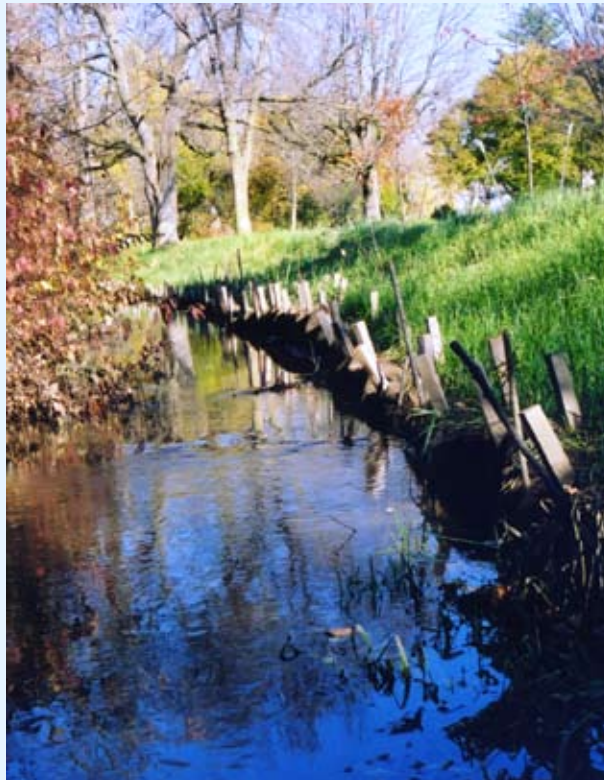
This creek has soft-engineering stabilization methods installed to protect the stream banks from erosion.
