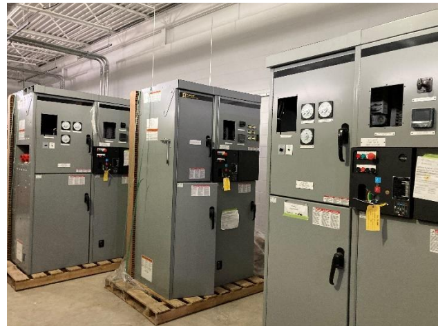
Additional electrical gear delivered to electrical building.
