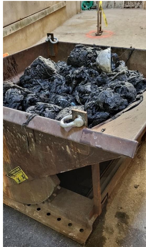
Ragging Removed from Bar Screens
