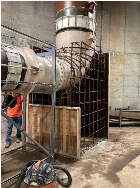
Forming Pump 1 Thrust Block
