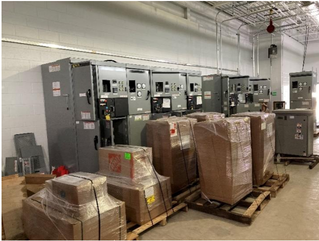
NESPS Electrical Room
