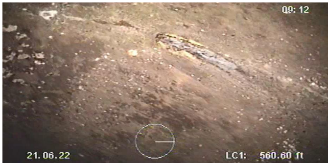
Infiltration Dripper between PCI-7-106 and PCI-7-107
