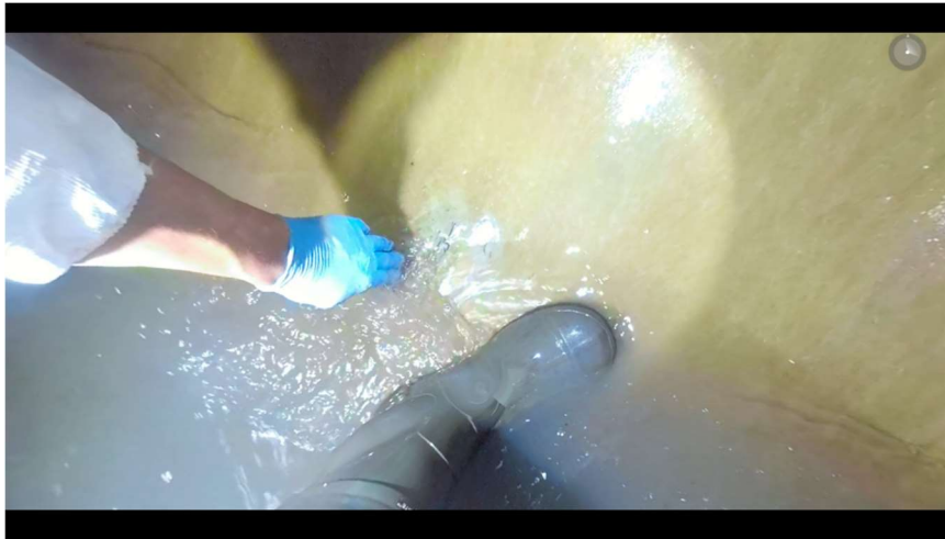
Photo 9: Damaged liner found at 855' downstream. Does not appear to be gouge from plate.
