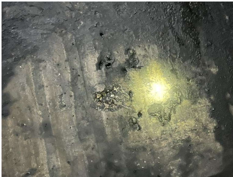
Photo 4: Spalled concrete on the east side of the shaft
