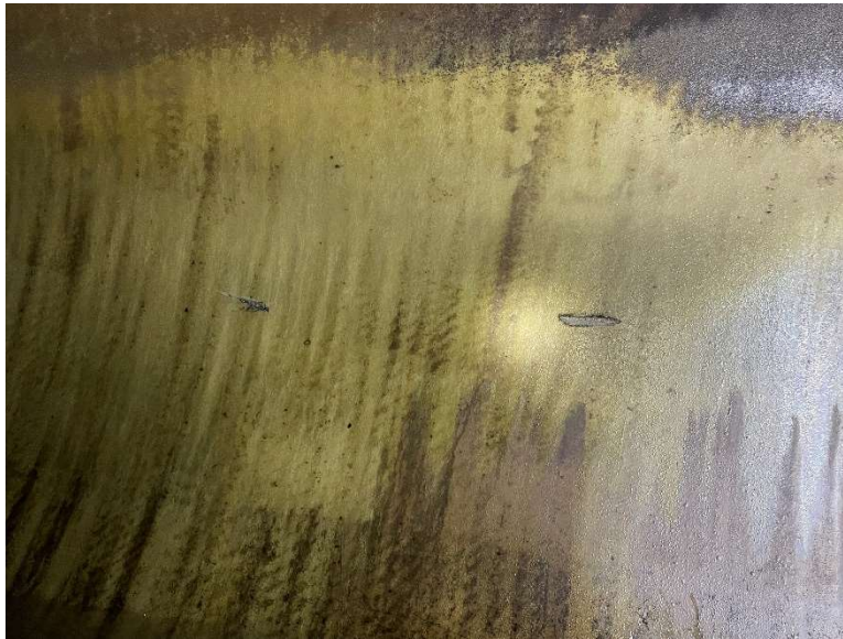
Photo 5: Gouges in liner at 5' and 6' downstream
