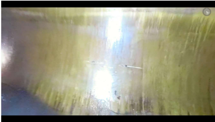
Photo 7: Gouges in liner at 24' and 25' downstream
