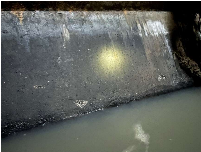
Photo 3: Spalled concrete on the west side of the shaft
