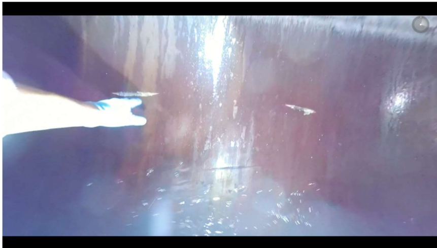
Photo 10: Gouges in liner at 1125' and 1126' downstream
