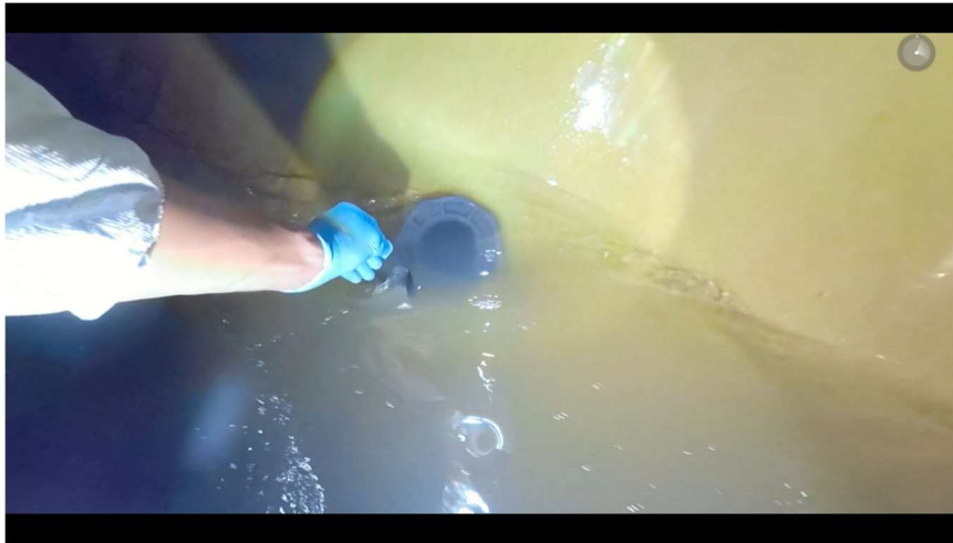
Photo 11: Damaged grout port at 684' downstream
