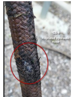
CS-9 Ruptured Hydraulic Hose
