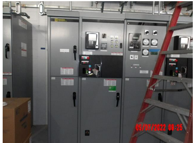
Electrical building motor control center switchgear. Location of arc flash incident.
