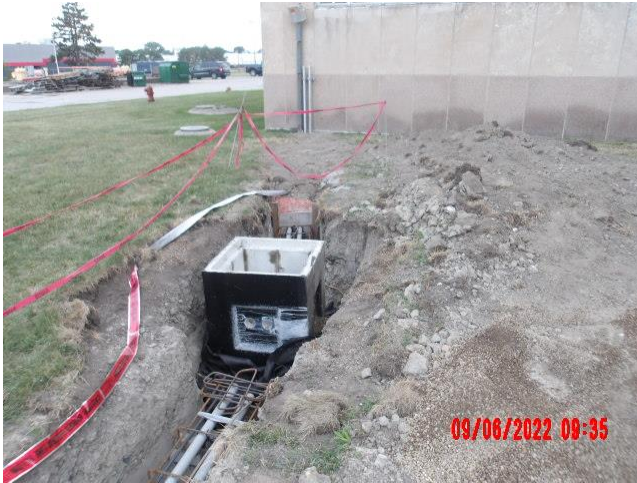
New fiber optic handhole
