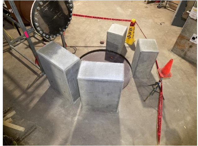
Pump #3 volute support foundations
