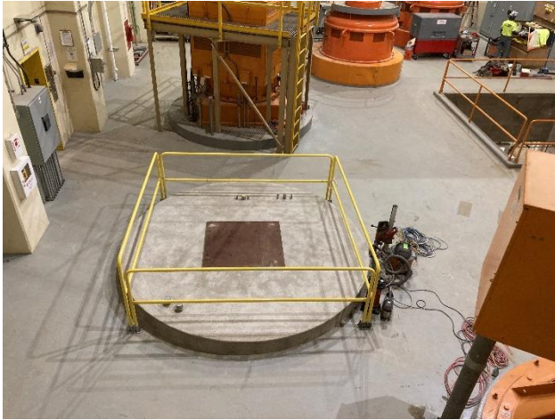
Pump #3 Motor Foundation Pad
