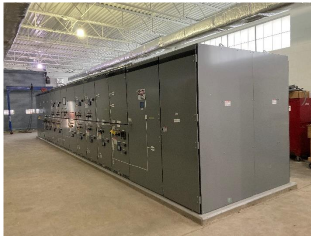
Metal-clad switchgear in the new electrical building
