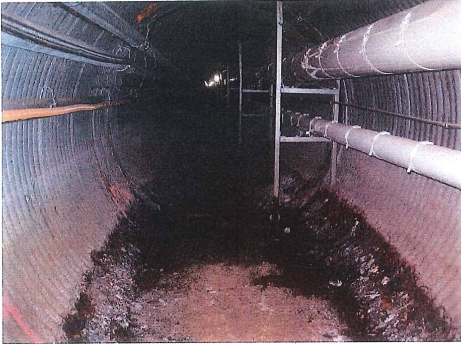
Fig. 5 Before – Sheriff Administration Steam Tunnel, north of County Center Drive, looking south. Electrical, communication and data cables on left side, supported by tunnel wall. Steam pipe, condensate pipe, electrical conduit on right side, supported by existing metal framing system.
