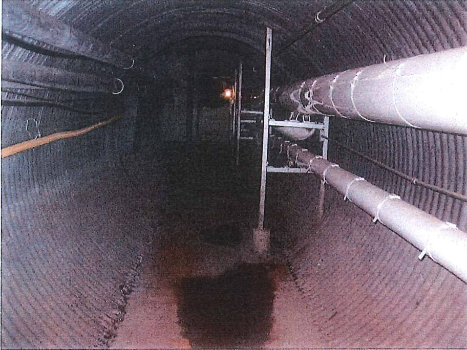
Fig. 4 Before – Sheriff Administration Steam Tunnel, north of creek, looking south. Electrical, communication and data cables on left side, supported by tunnel wall. Steam pipe, condensate pipe, electrical conduit on right side, supported by existing metal framing system.
