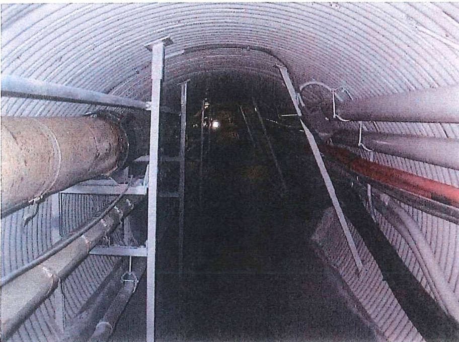
Fig. 2 After – Resource & Crisis Center Steam Tunnel, under building, looking north. Electrical, communication and data cables on right side, supported by new brackets. New tunnel coating and structural floor.
