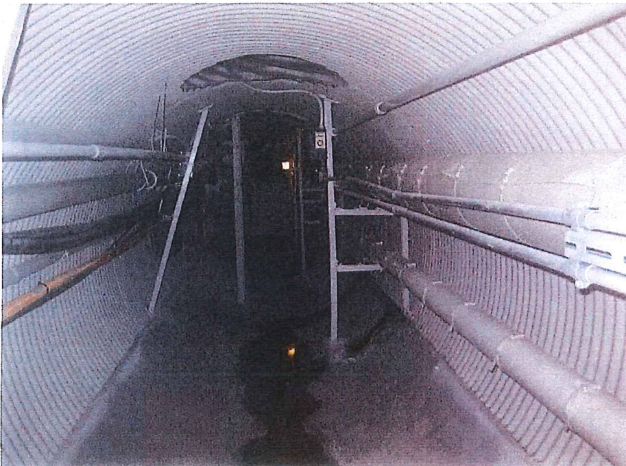
Fig. 4 After – Sheriff Administration Steam Tunnel, north of creek, looking south. Electrical, communication and data cables on left side, supported by new brackets. New tunnel coating, exhaust fan and structural floor.
