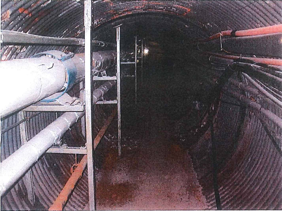
Fig. 2 Before – Resource & Crisis Center Steam Tunnel, under building, looking north. Electrical, communication and data cables on right side, supported by tunnel wall. Steam pipe, condensate pipe, electrical conduit on left side, supported by existing metal framing system.
