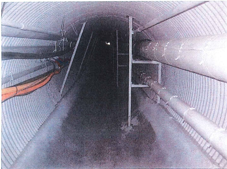
Fig. 5 Before – Sheriff Administration Steam Tunnel, north of County Center Drive, looking south. Electrical, communication and data cables on left side, supported by new brackets. New tunnel coating and structural floor.
