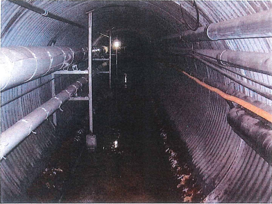
Fig. 3 Before – Resource & Crisis Center Steam Tunnel, north of building, near creek, looking north. Electrical, communication and data cables on right side, supported by tunnel wall. Steam pipe, condensate pipe, electrical conduit on left side, supported by existing metal framing system.
