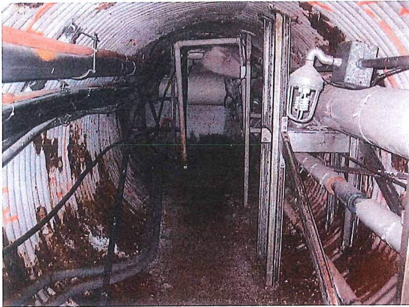
Fig. 1 Before – Resource & Crisis Center Steam Tunnel, south edge of building, looking south. Electrical, communication and data cables on left side, supported by tunnel wall. Steam pipe, condensate pipe, electrical conduit on right side, supported by existing metal framing system.
